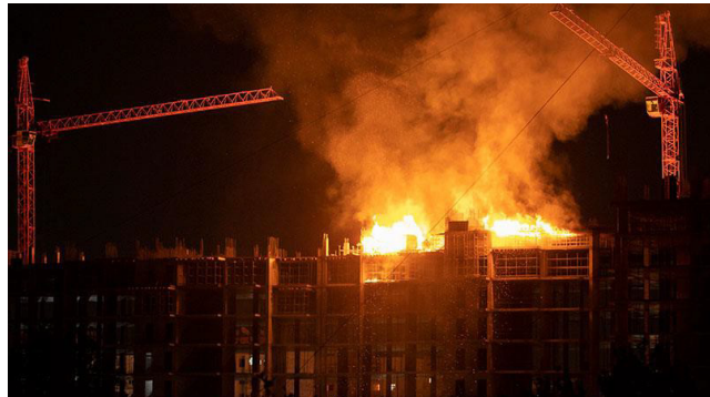
Fig. 7.2.3 Fire at Construction Site
