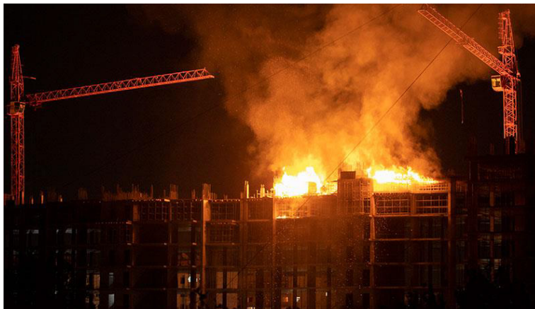
Fig. 5.2.3 Fire at Construction Site
