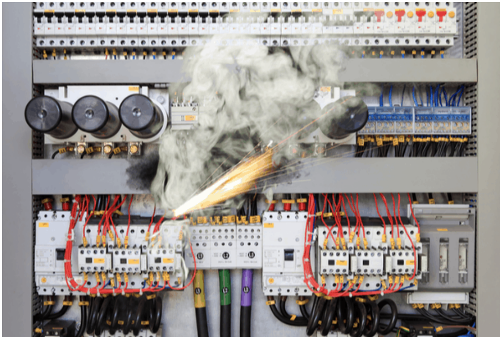
Fig. 5.2.1: Faults in temporary electrical panels
