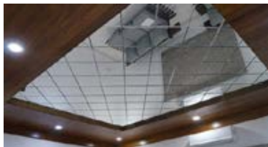
Fig. 4.1.8 Glass False Ceiling
