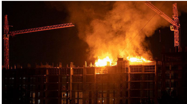
Fig. 10.2.3 Fire at Construction Site
