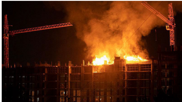
Fig. 7.2.3 Fire at Construction Site
