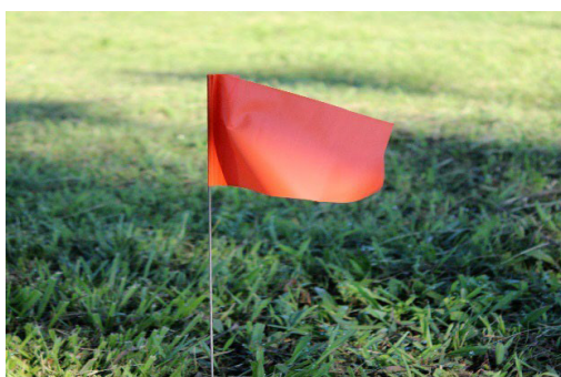
Step 5: Have all marking tools like lime, wooden pegs, rope, flag, etc. ready.
