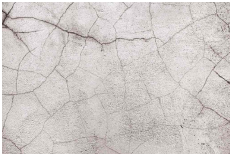
Fig. 6.2.1 Improperly cured concrete surface
