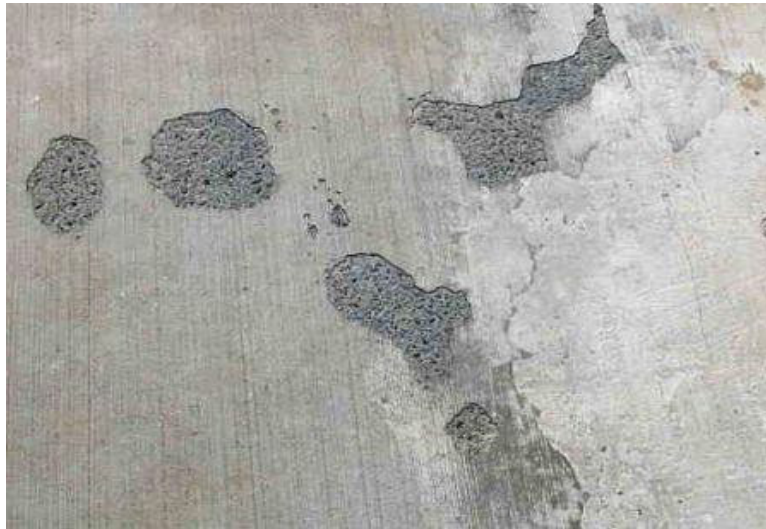
Fig. 3.5.2 Defect in concrete structure
