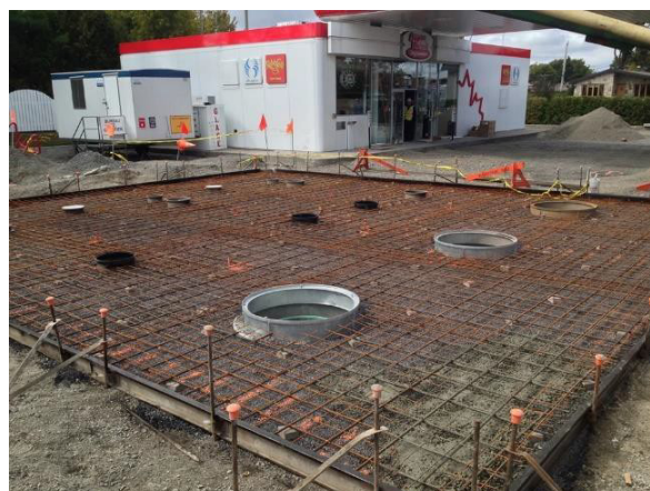
Fig. 4.1.9 Wire mesh used for reinforcement
