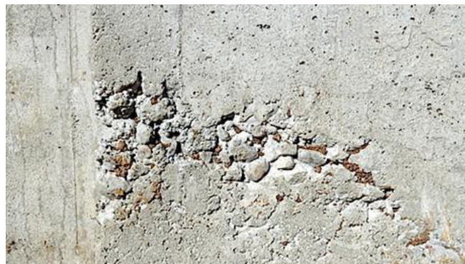
Fig. 3.5.1 Defect in concrete structure due to honeycombing
