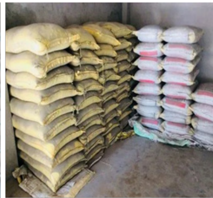
3.1.7 Wrong Way of Keeping Cement
