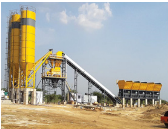
Fig. 1.3.5 Batching Plant for Concrete Mixing
