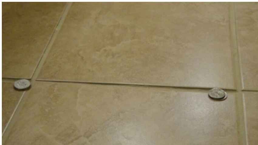
Fig. 5.2.4 Uneven Tiles and Lippage Issue
