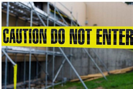
Step 7: Barricade the area using fencing or barricade materials and place safety signage.
