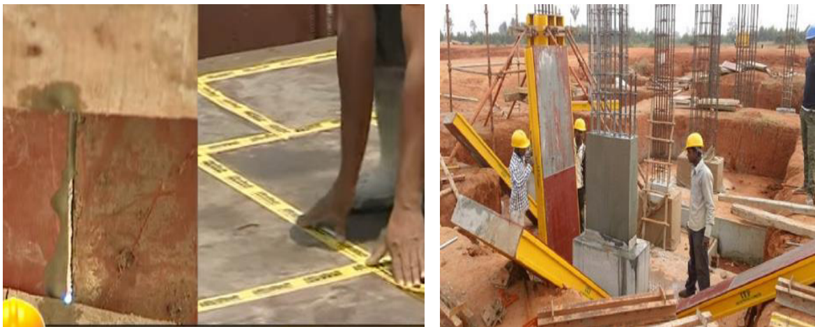
Fig 9.2.18: Covering airgap by tape
